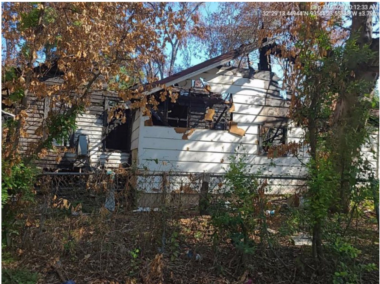
Exhibit D. - Fire Damaged Property Conditions
