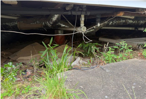
Live wire tied around sewer pipe
