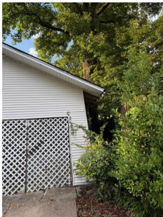
Garage sites on western property line; also has a mature tree growing out of it
