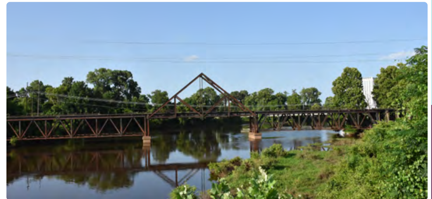
The historic A-Truss bridge over Twelve Mile Bayou can connect future pedestrians and cyclists on a future Cross Bayou greenway and blueway. Source: Asakura Robinson
