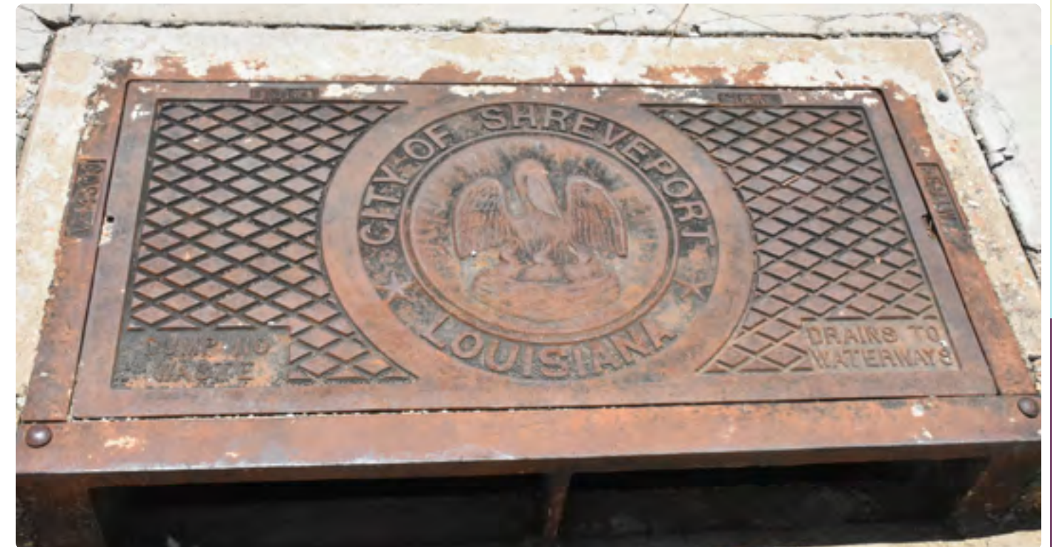
This stormwater inlet reminds users to “dump no waste” and that stormwater “drains to waterways”. Source: Asakura Robinson
